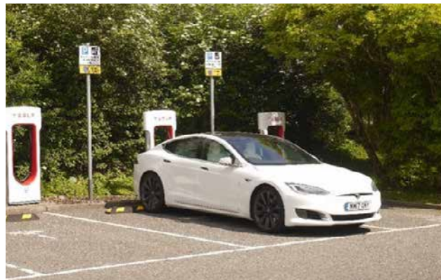
Figure 57: Example of electric vehicle charging points in a parking court.
